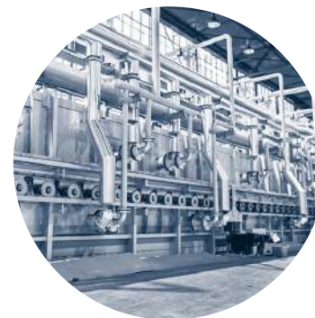
New steel heat treatment line, SIJ Metal Ravne
